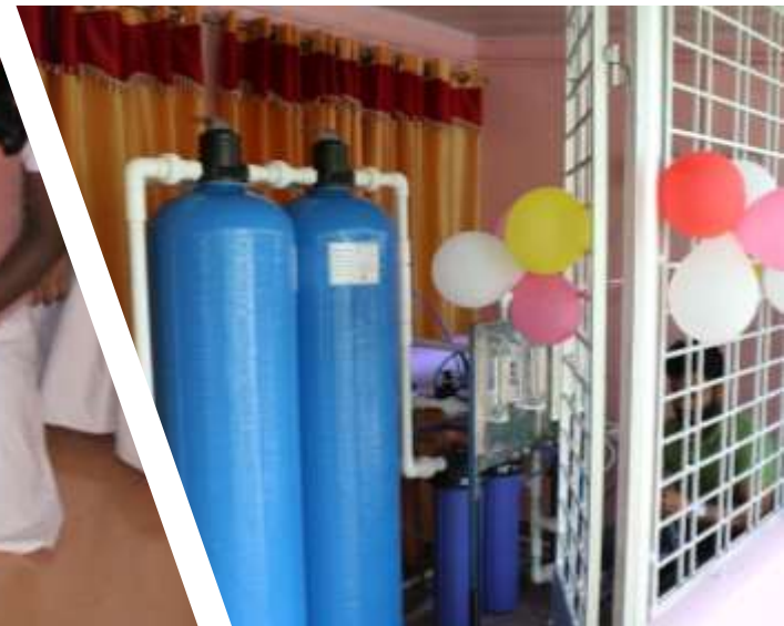
Installed RO plant in Kainakary, Alappuzha
